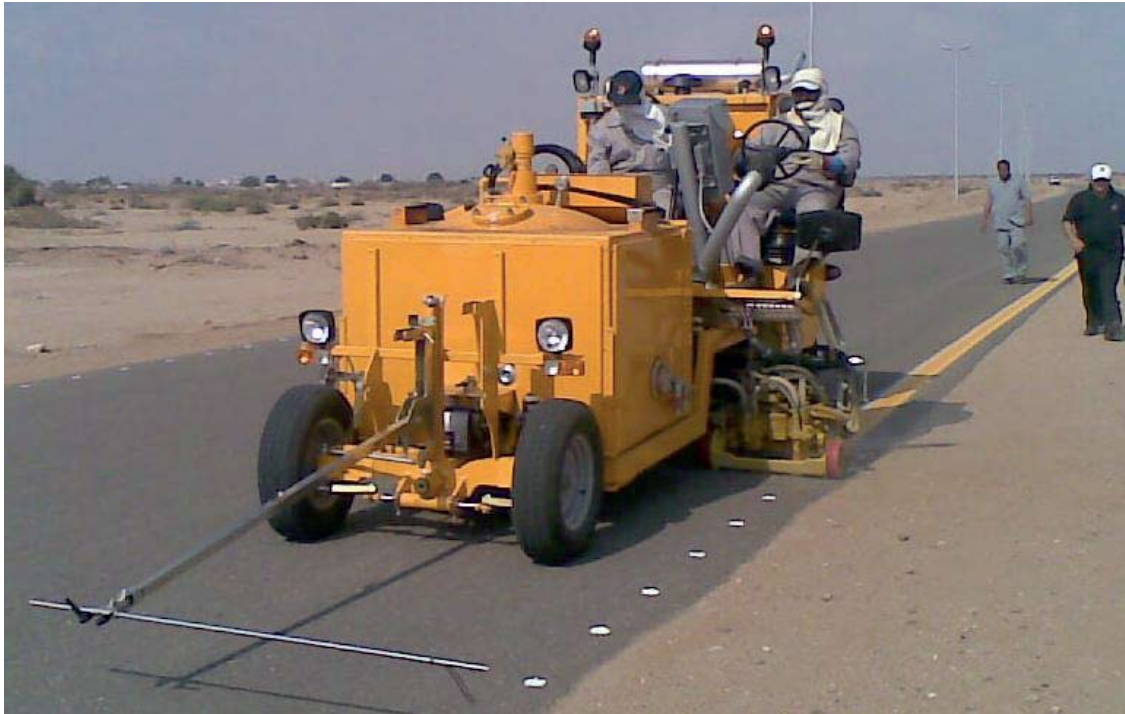
Following a brief training period with the Borum service team, Al Owaidah has now concluded an impressive road marking project in Jizan, close to the Saudi Arabia-Yemen border.
