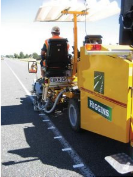
Higgins' Borum BMT 350 road marking machine at work on SH 1 on New Zealand's North Island
